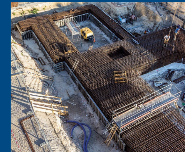
The tower's base area before the foundation plate was cast, photo: Dr. Peter-M. Bauers
